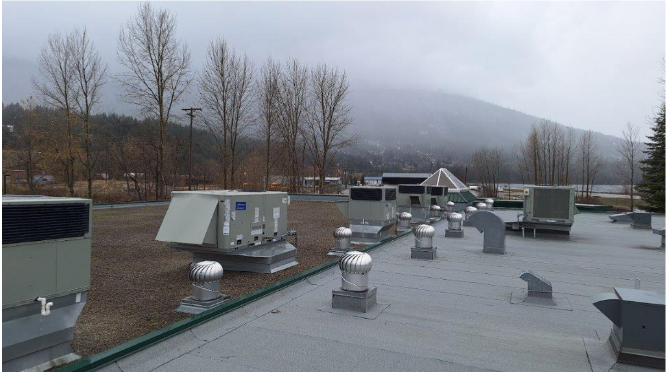
Separation between old and new sections of roof
