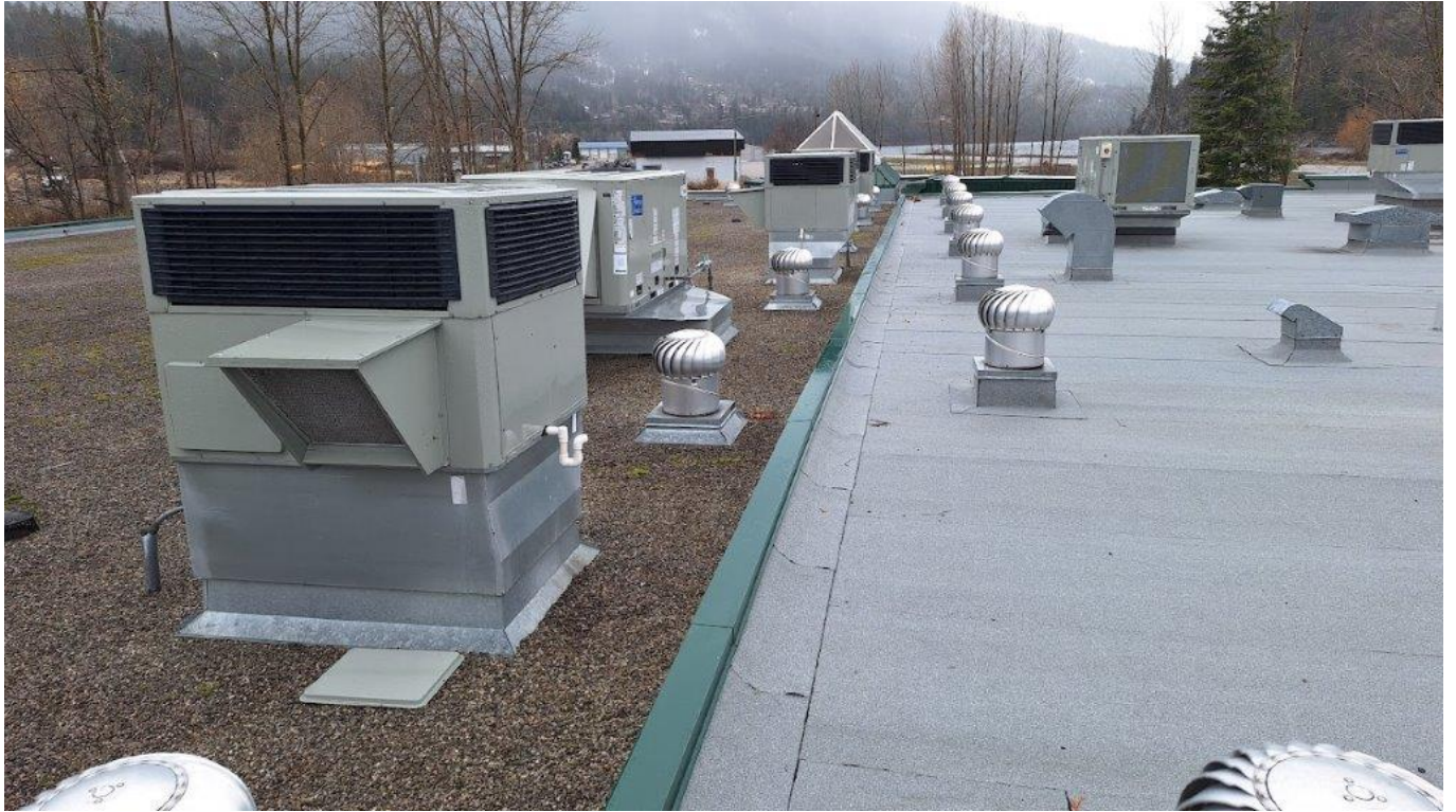
Separation between old and new sections of roof – all roof top units and curbs have been replaced in 2022
